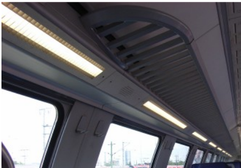
Application example of a 110 V LED tube in subways
