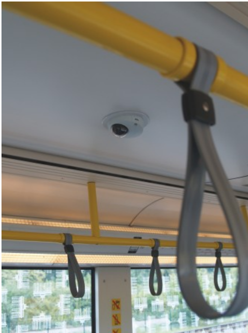
IP-cameras monitor different places in public transport e.g. platforms
